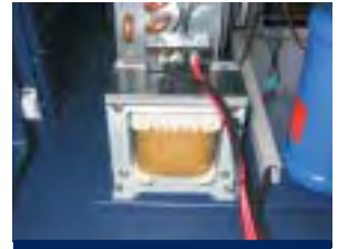
Automatic voltage compensation protects electrical components
